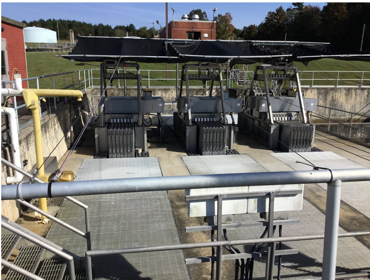
UV System at the Eastside WWTP
