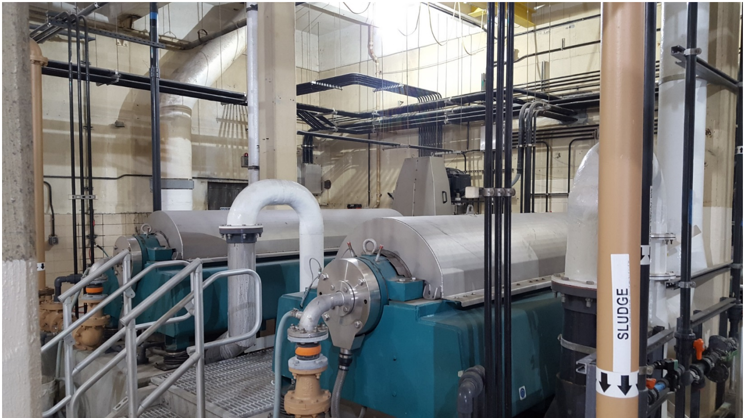
Eastside WWTP Centrifuges 1 and 2
