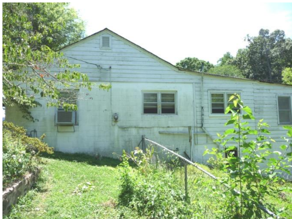
Before lead hazard remediation...
