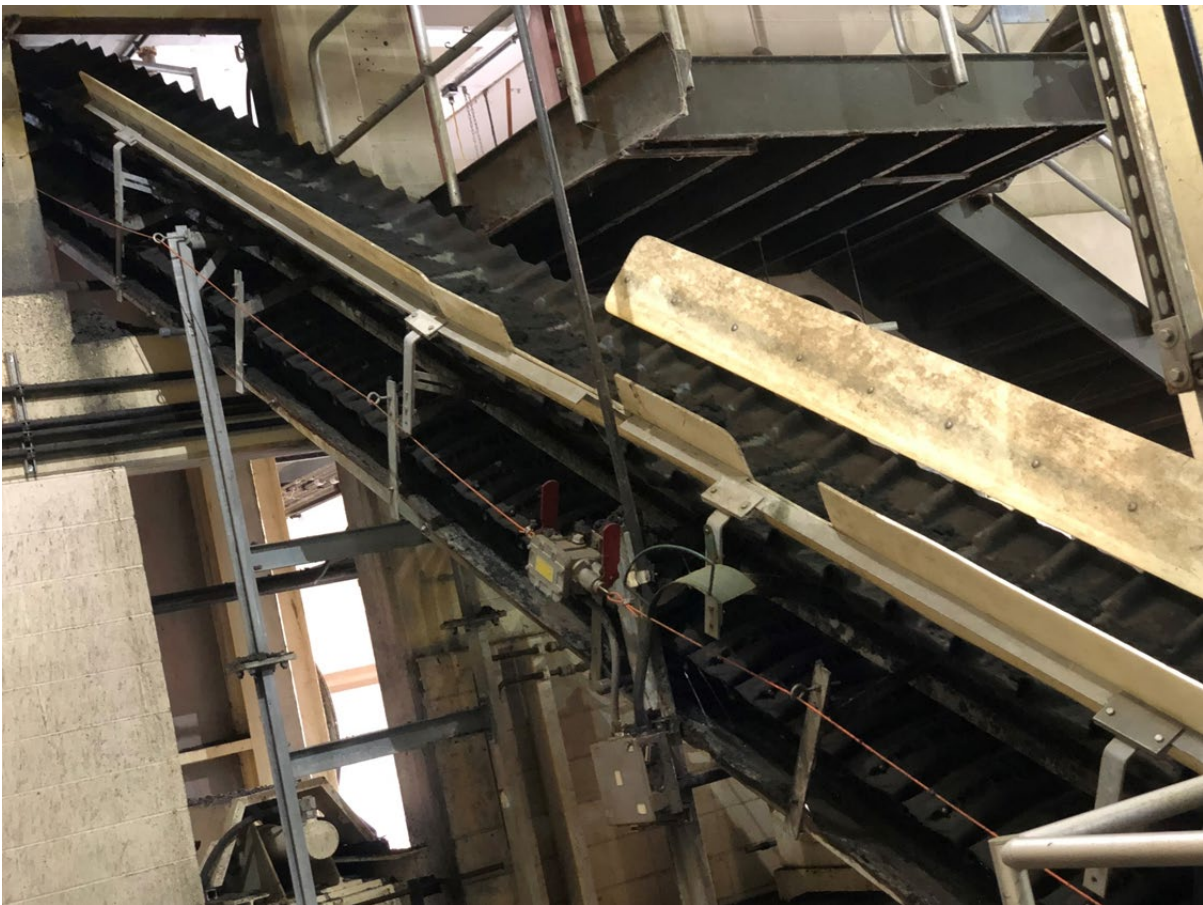
Serpentix Conveyor at the Eastside WWTP
