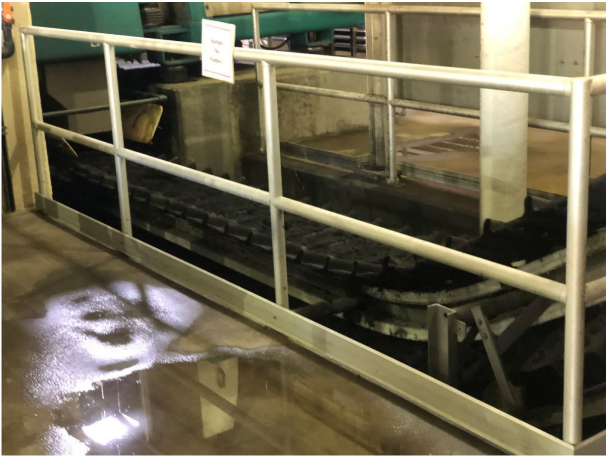
Serpentix Conveyor at the Eastside WWTP
