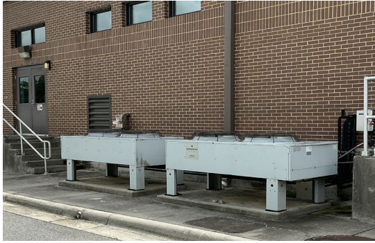
Liebert Condensers- Filter Building
