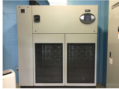
Liebert Air Handling Unit- Filter Building
