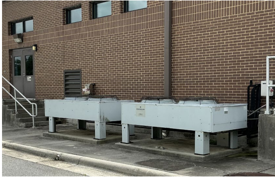
Liebert Condensers- Filter Building
