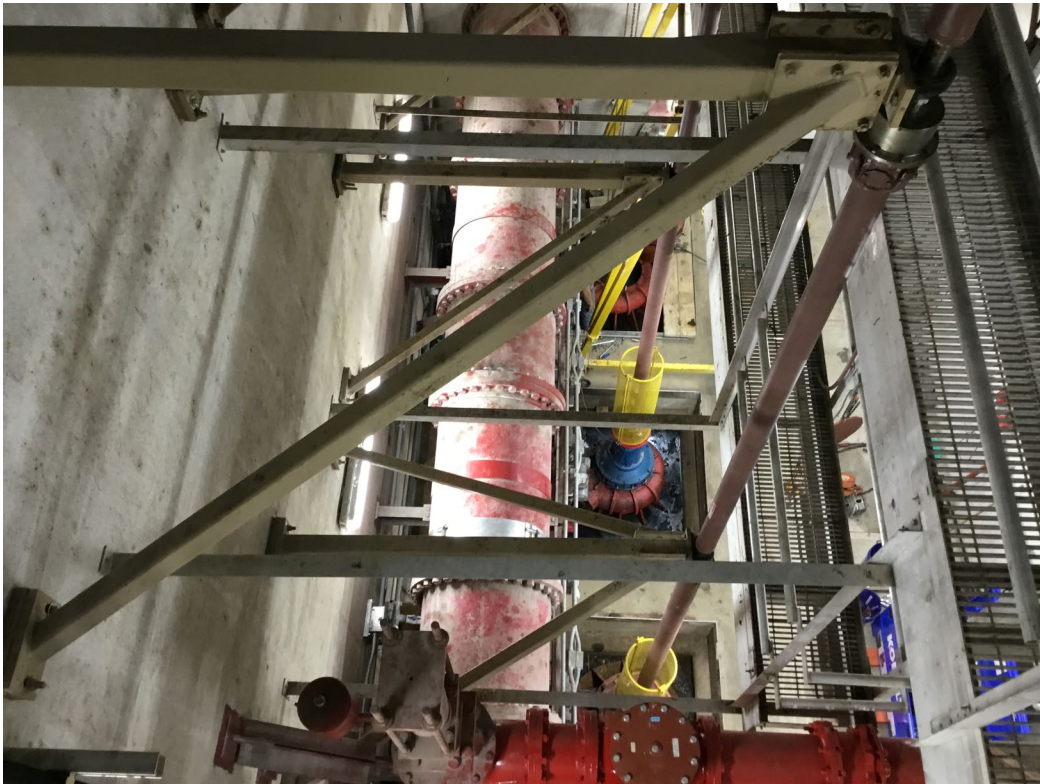
Picture of the 3 screw centrifugal pumps and drive shafts in the Riverdale Pump Station dry well.
