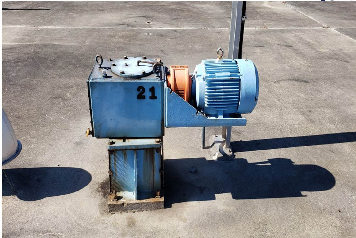
Example of a Gear Box at the Eastside WWTP
