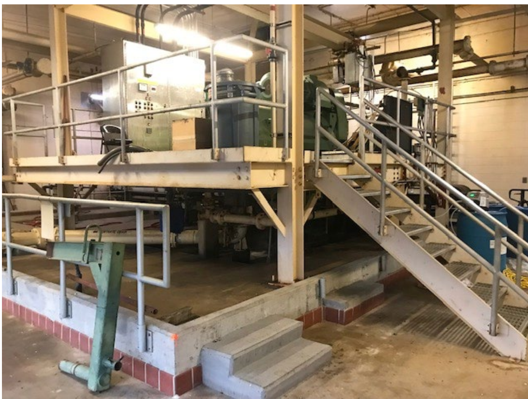
Platform for existing centrifuge and controls.
