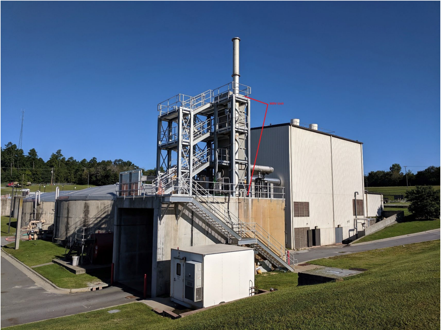
Incinerator stack with MRV unit identified with red lines.
