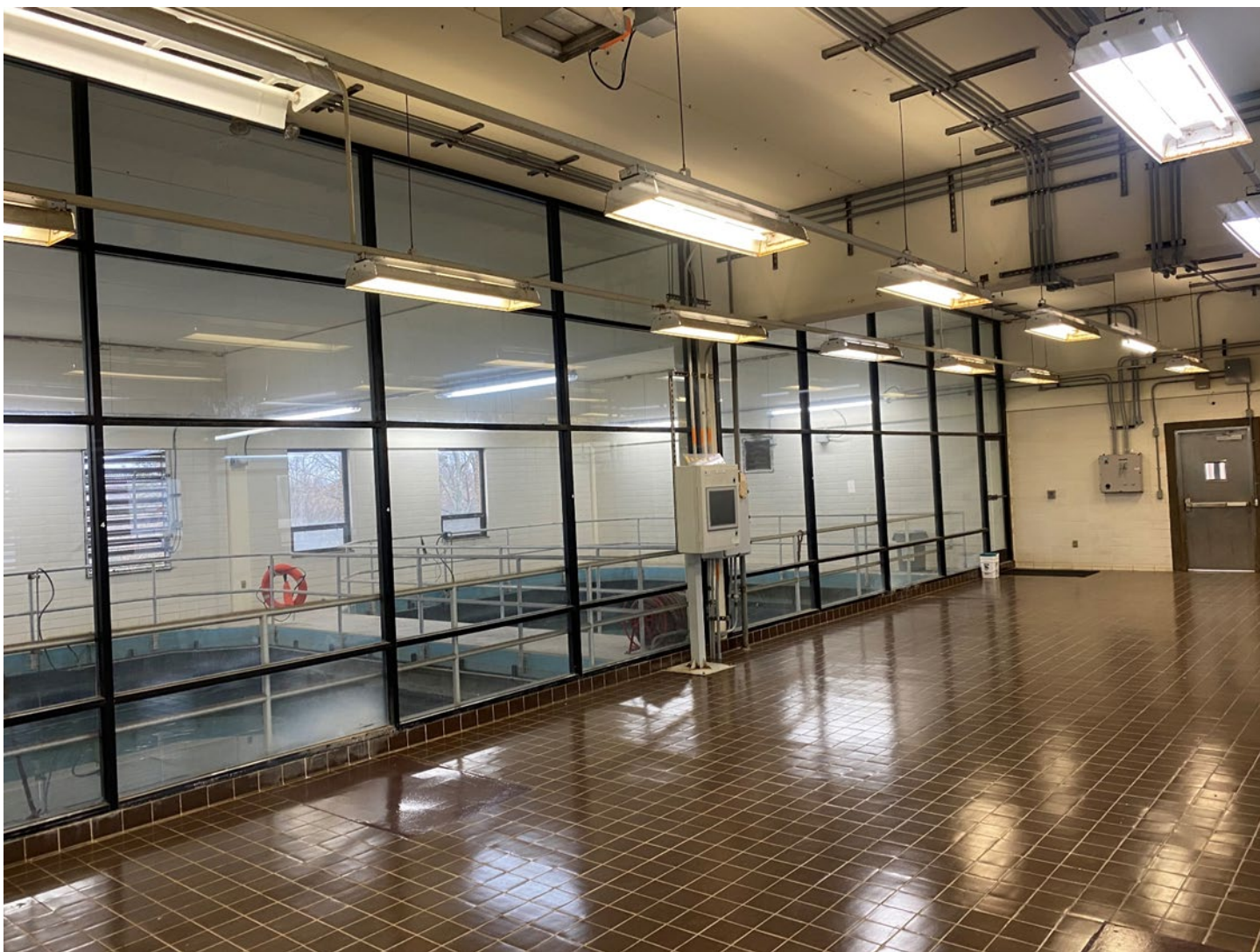
Ward WTP Filter Room
