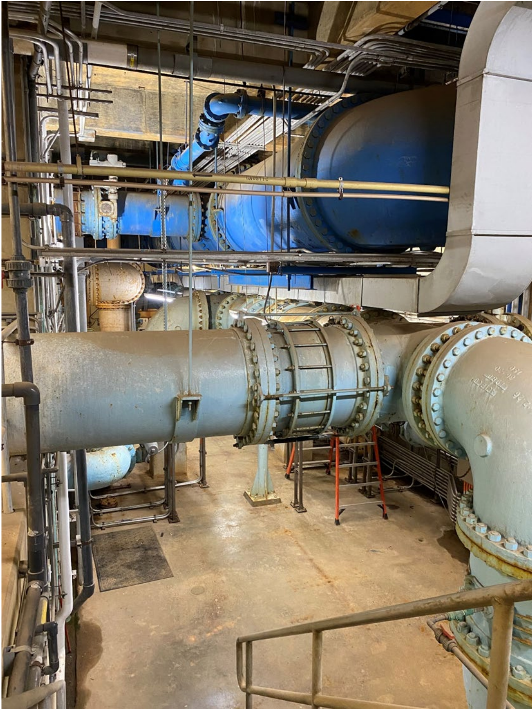
Ward WTP Pipe Gallery
