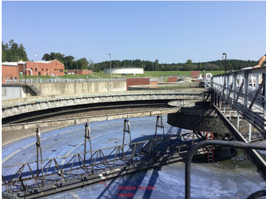
View of a drained final clarifier
