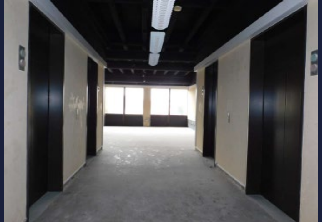
Upper Level Elevators
