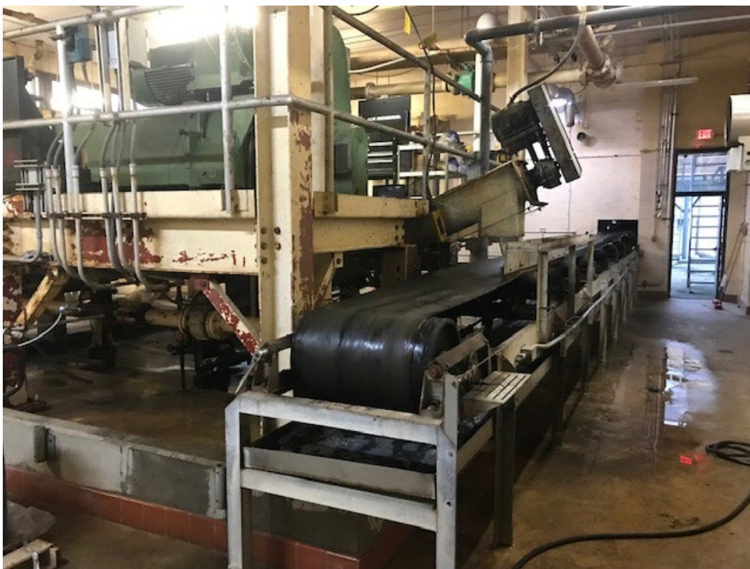
Existing inclined screw conveyor and conveyor that carries solids to the loading area
