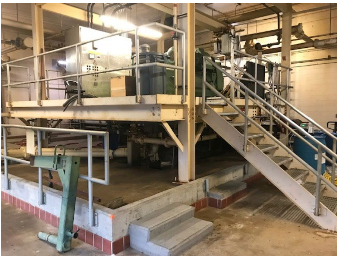
Platform for existing centrifuge and controls.
