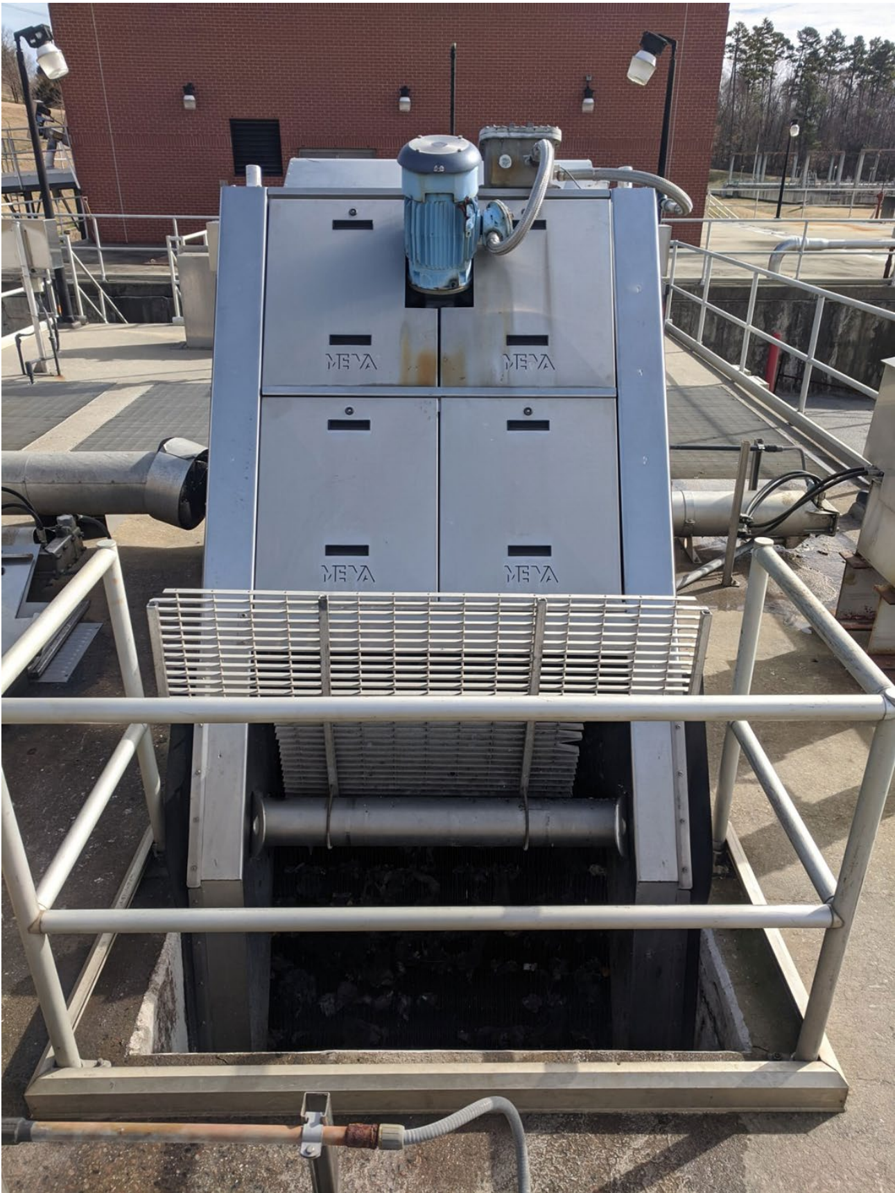
Example Bar Screen at the Eastside WWTP
