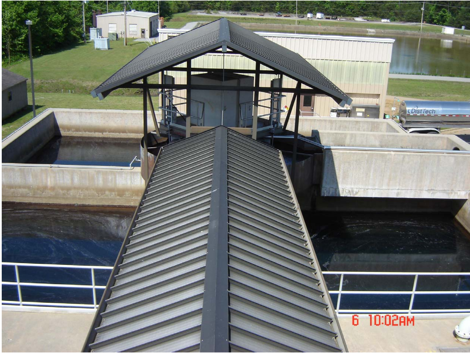
Looking down onto Filters 5-8
