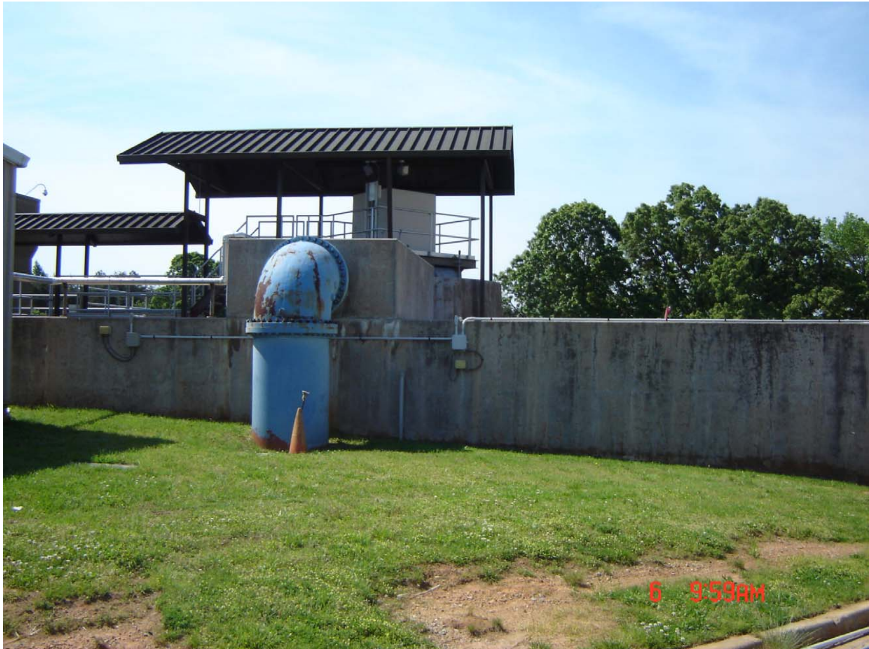
Exterior View – Filters 5-8
