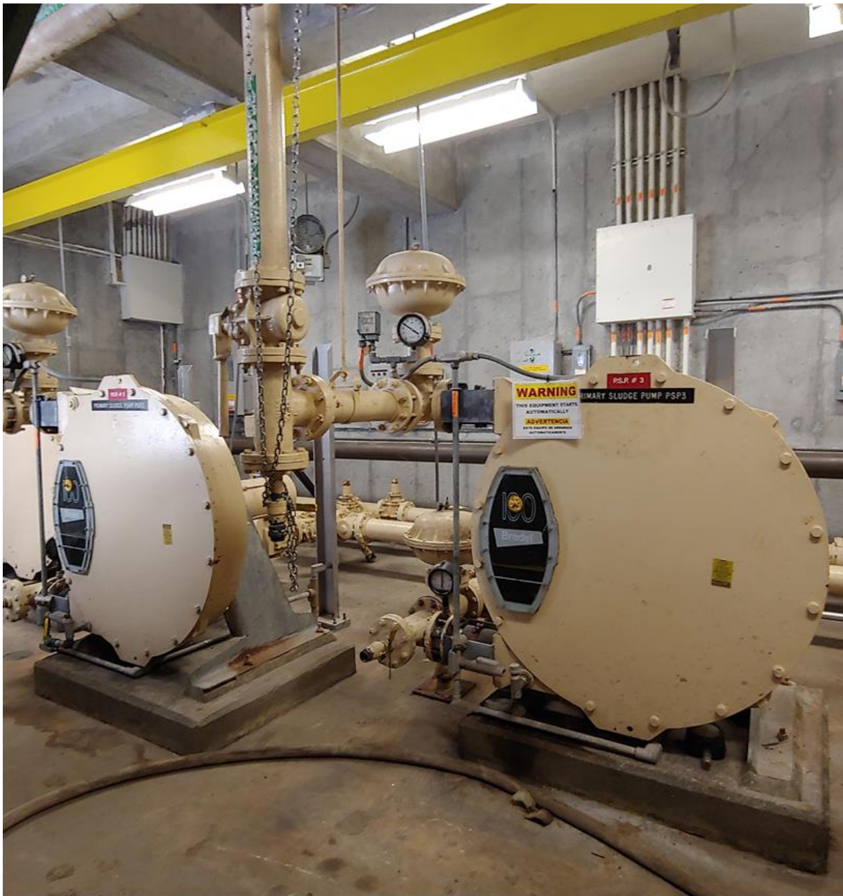
Existing Primary Sludge Peristaltic Pumps
