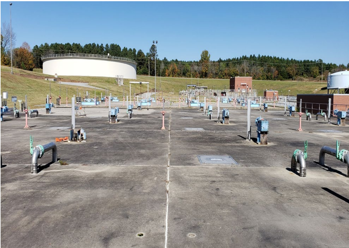
Gear Boxes on top of the AAA tanks at the Eastside WWTP
