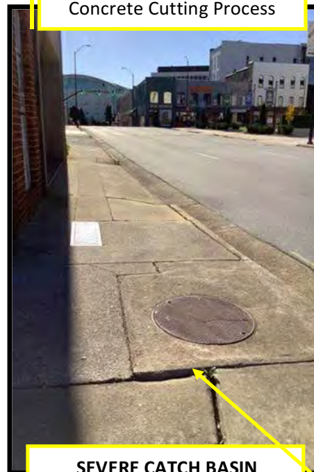
SEVERE CATCH BASIN TRIP AND FALL HAZARD Repairable using Precision Concrete Cutting Process
