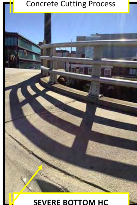
SEVERE BOTTOM HC TRIP AND FALL HAZARD Repairable using Precision Concrete Cutting Process
