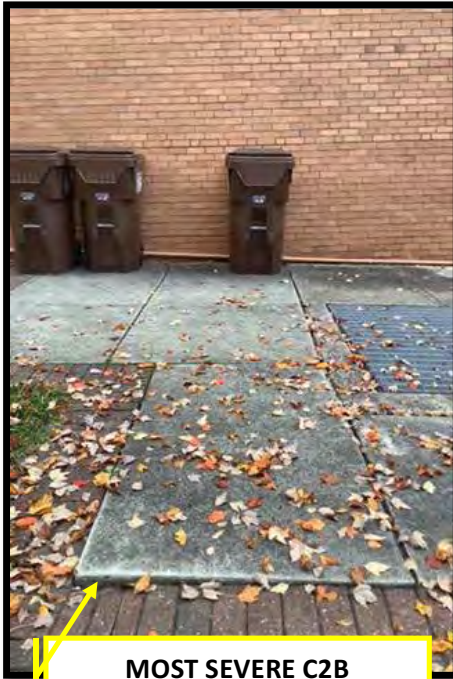
MOST SEVERE C2B TRIP AND FALL HAZARD Repairable using Precision Concrete Cutting Process
