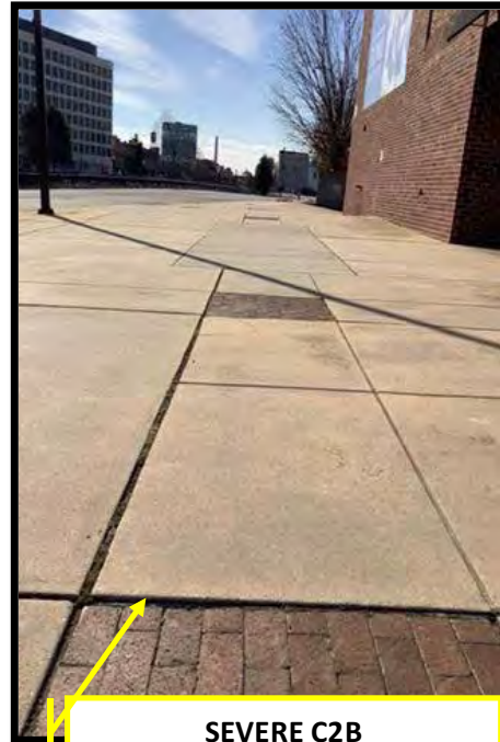
SEVERE C2B TRIP AND FALL HAZARD Repairable using Precision Concrete Cutting Process
