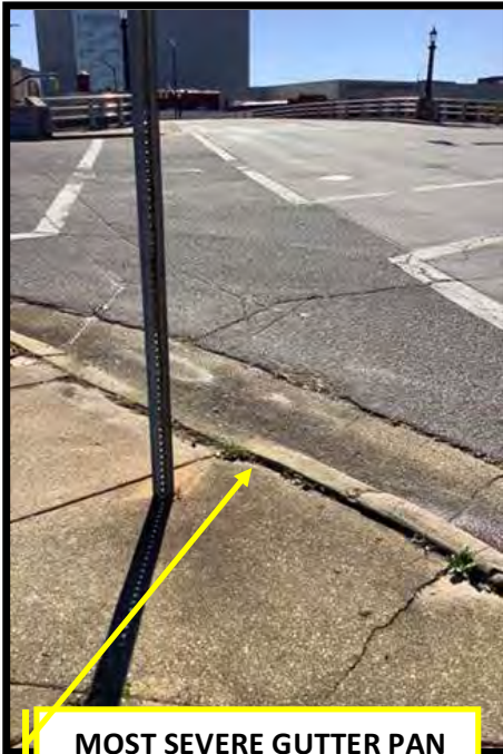
MOST SEVERE GUTTER PAN TRIP AND FALL HAZARD Repairable using Precision Concrete Cutting Process
