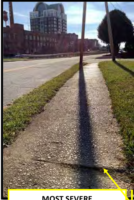
MOST SEVERE TRIP AND FALL HAZARD Repairable using Precision Concrete Cutting Process
