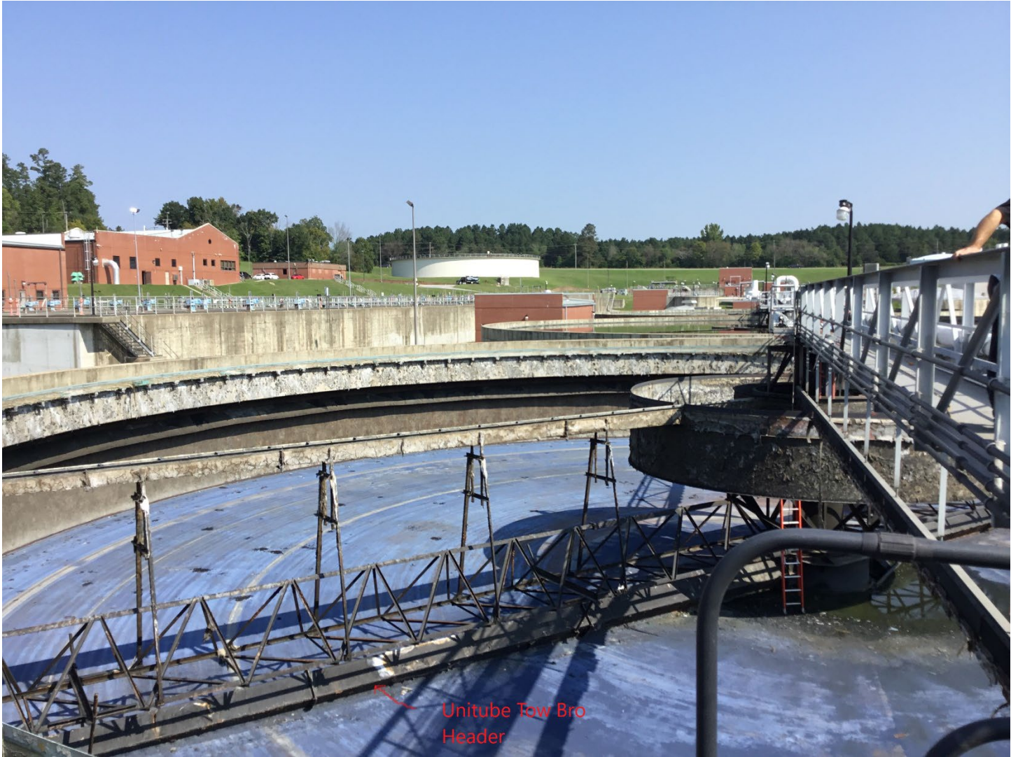
Final Clarifier #3 Drained.
