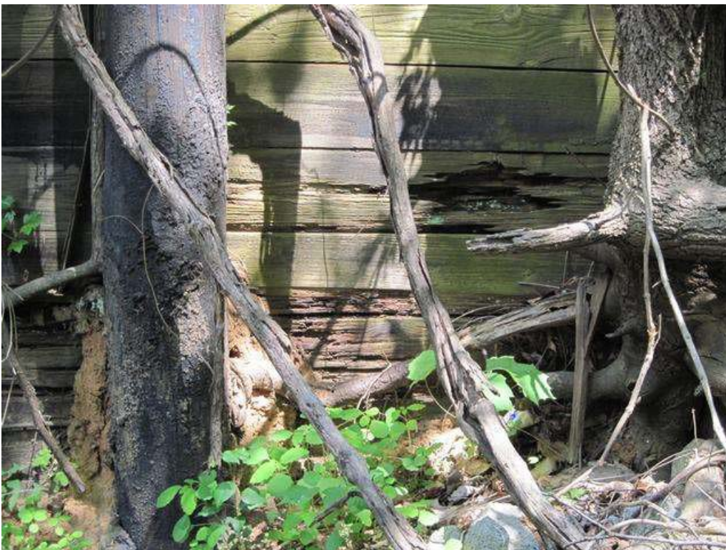
Decaying boards on the southeast wingwall.
