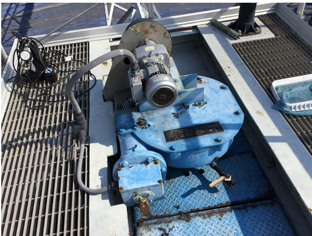
Top view of existing drive unit.
