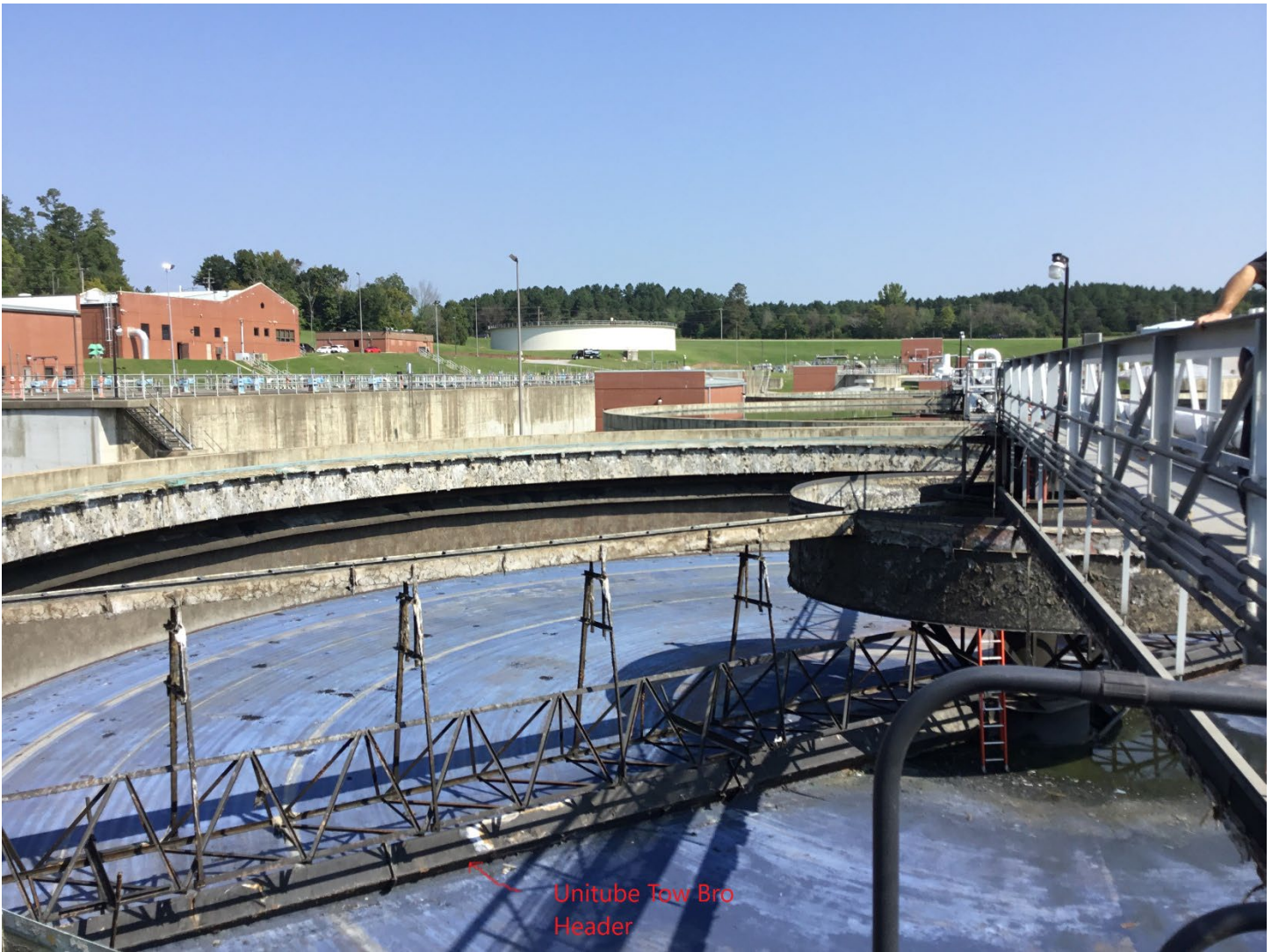
Final Clarifier #3 Drained.
