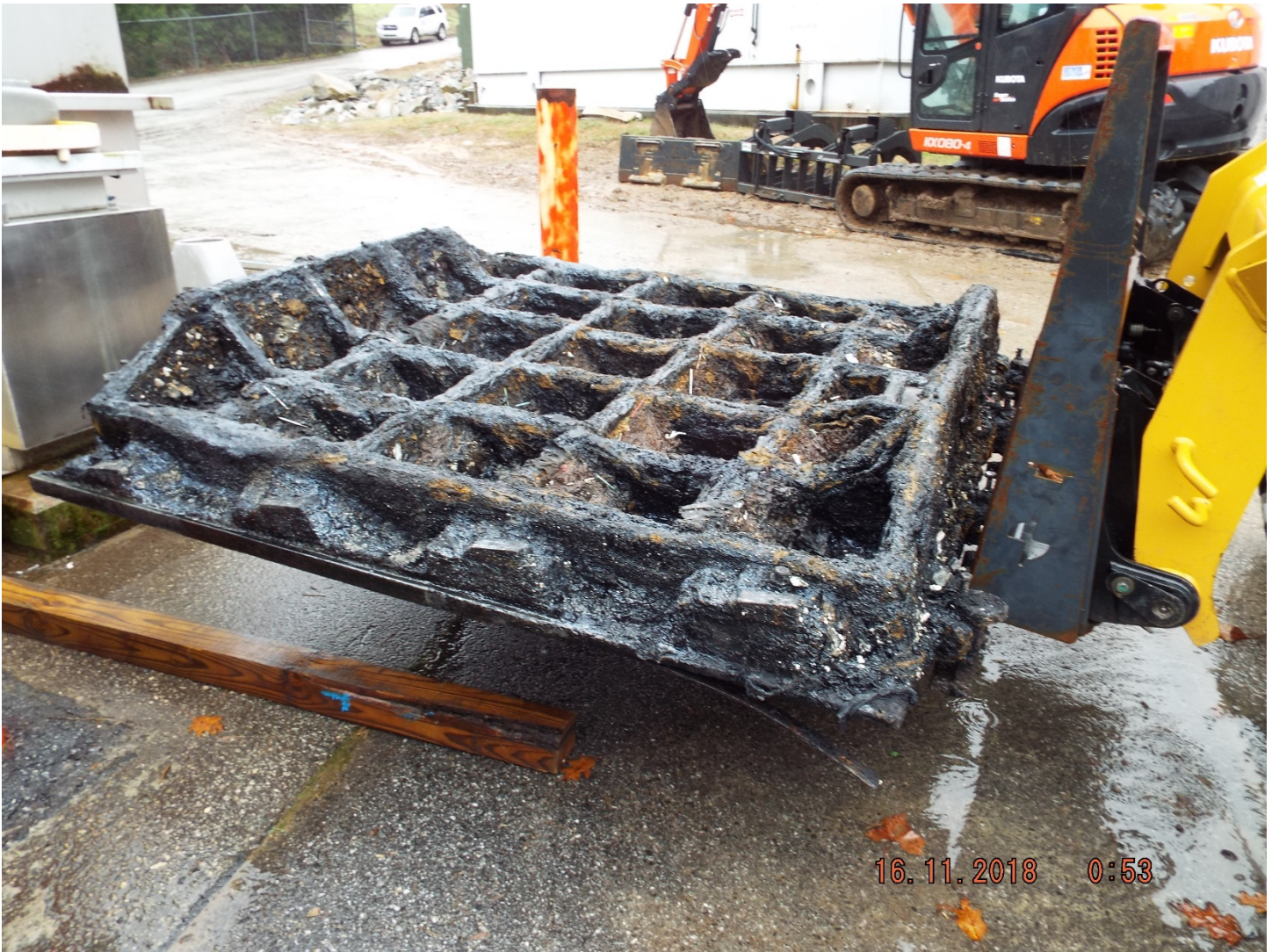
Deteriorated Sluice Gate
