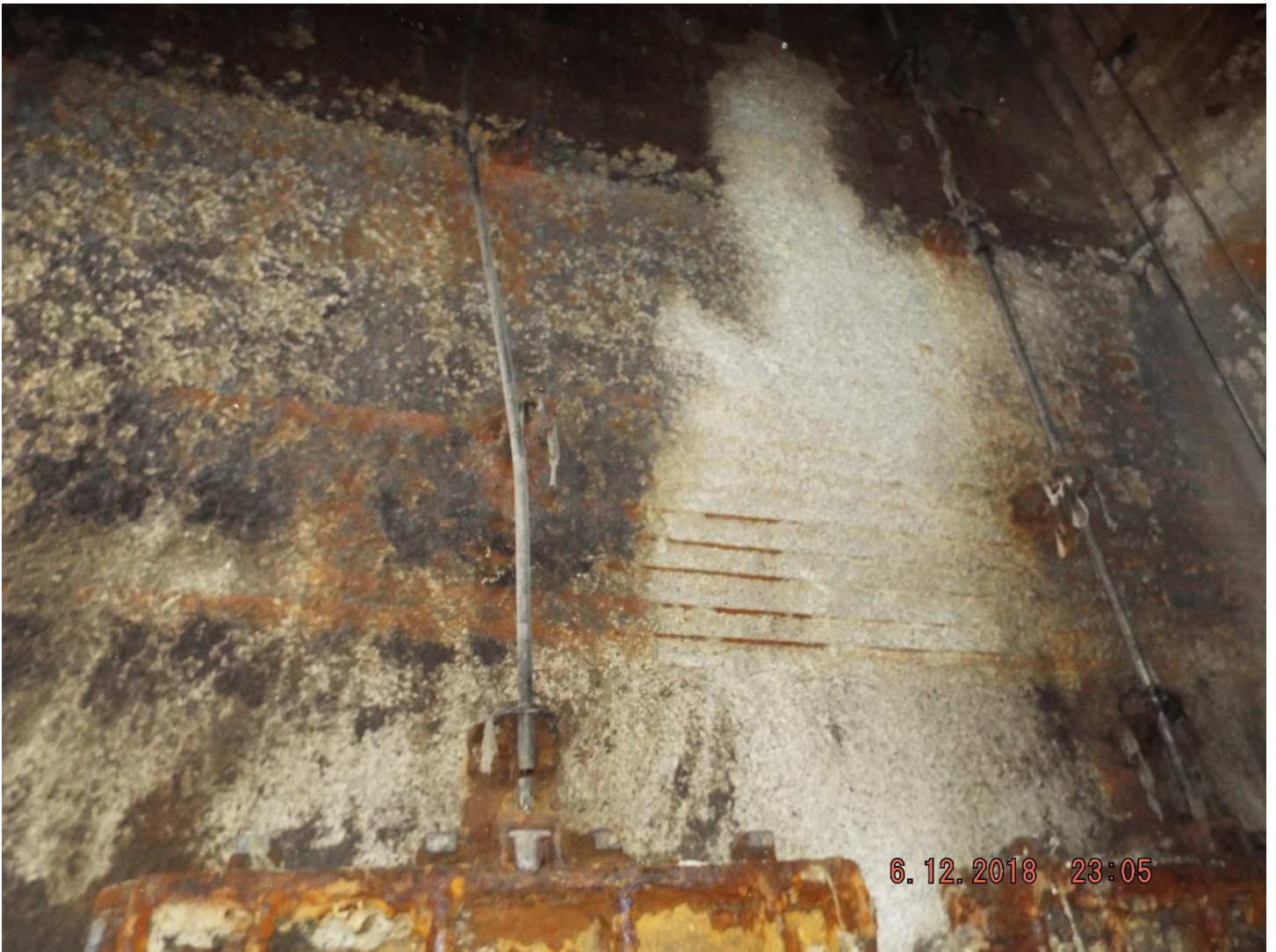
Deterioration of Wet Well Walls
