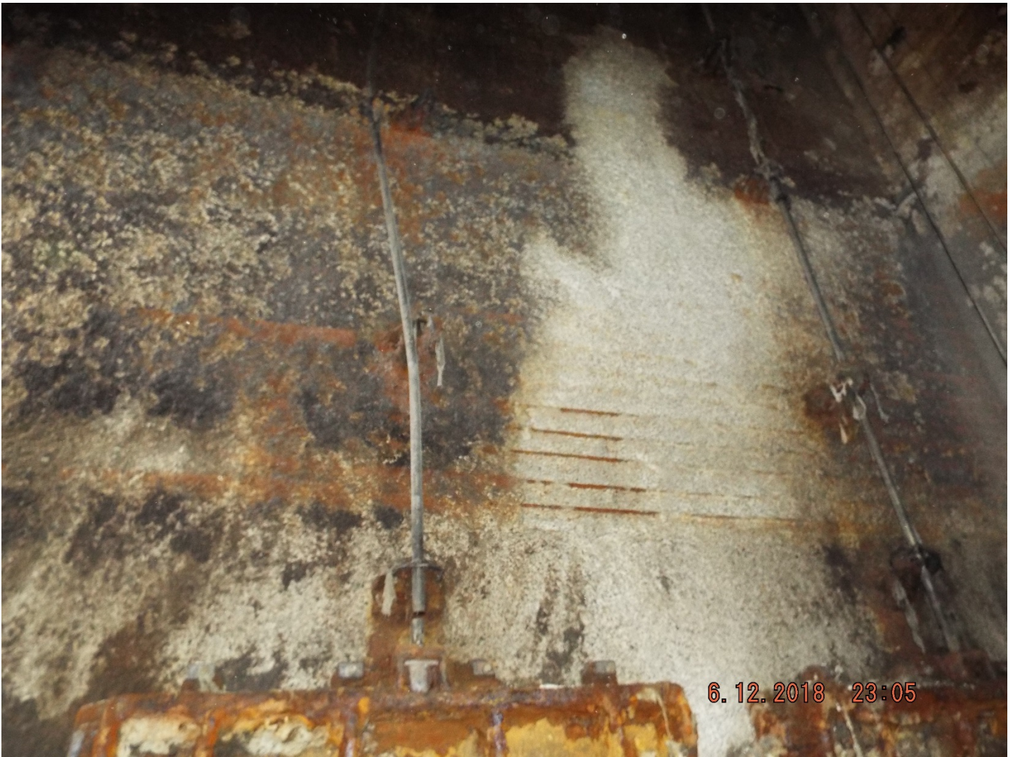
Deterioration of Wet Well Walls
