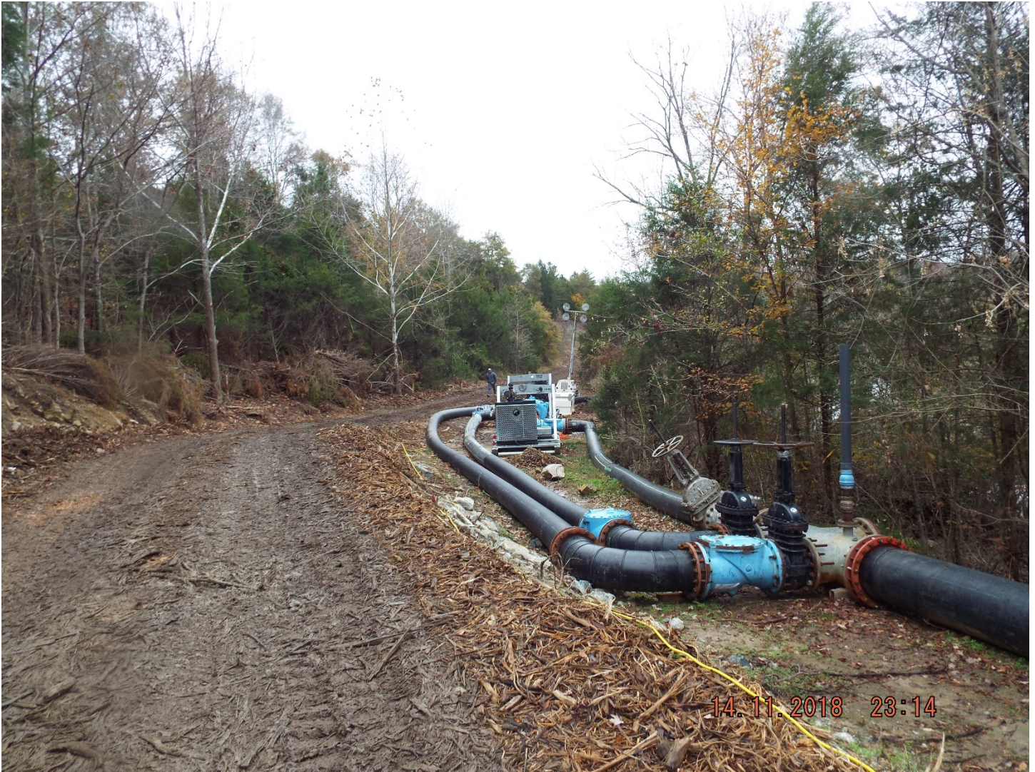
Picture of Emergency Bypass
