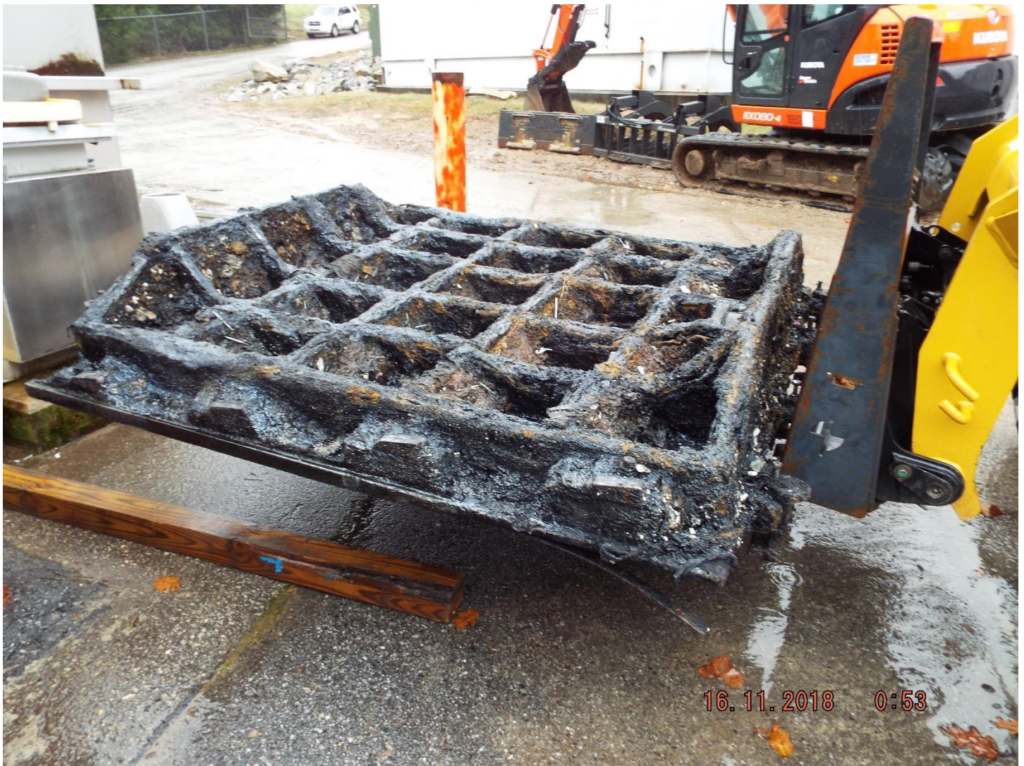
Deteriorated Sluice Gate
