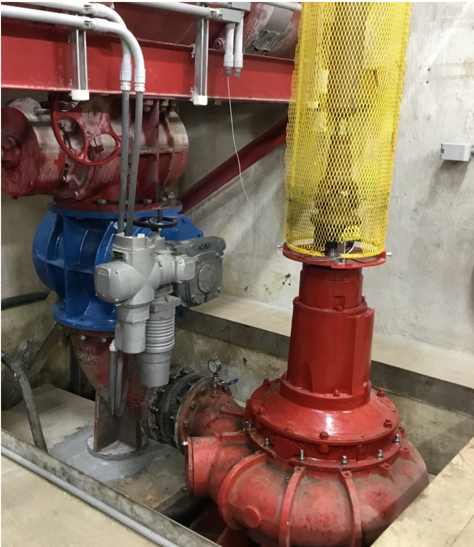
Picture of a Wemco-Hidrostal Pump in the Riverdale Pump Station
